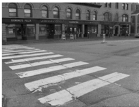
Some pedestrians complain that crosswalk signs are not visible enough for drivers to see
